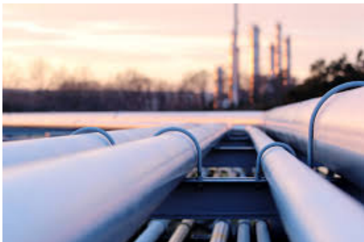
Pipelines & Fossil Fuel Infrastructure n= 38
